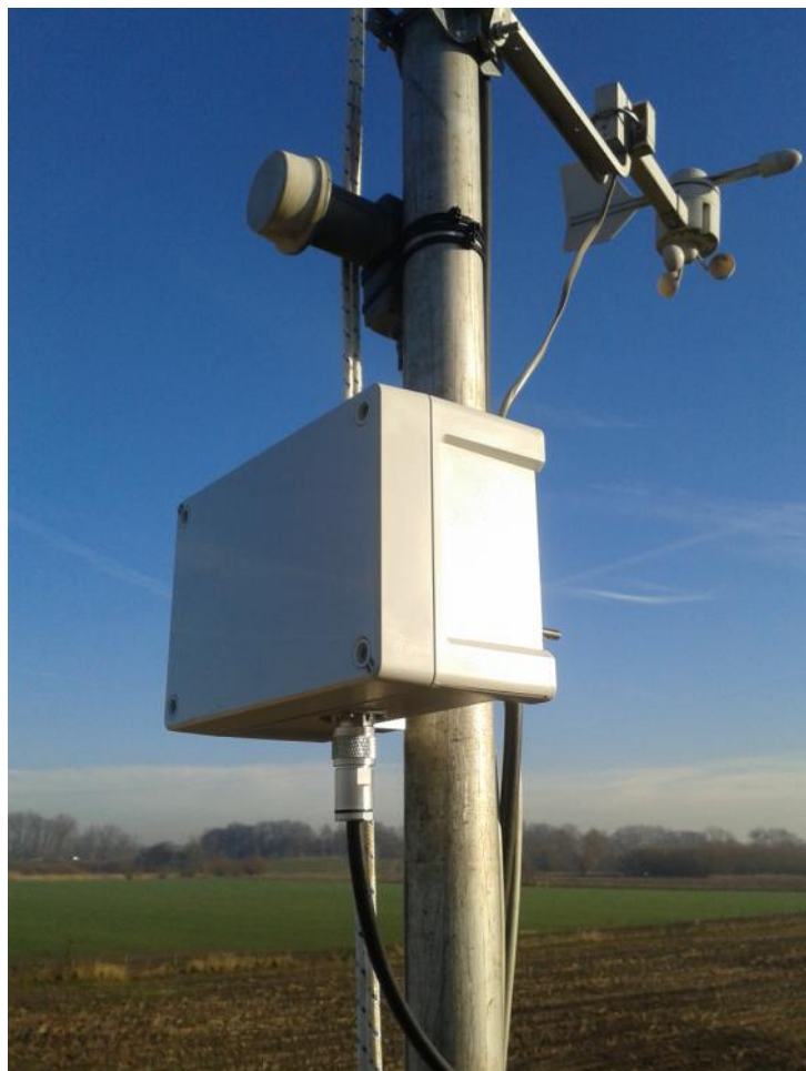
The antenna mounted in my pole, just below the 3cm LNC. Both are pointing at the PI6ATV repeater.
